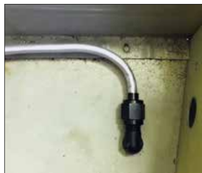
Vent line 90-degree bulkhead fitting pass-through on the bottom of the fuselage.
