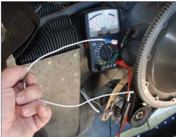
It can be quite difficult to access some field connections on alternators installed in airplanes. Here a pigtail has been made to make checking resistance easier.
