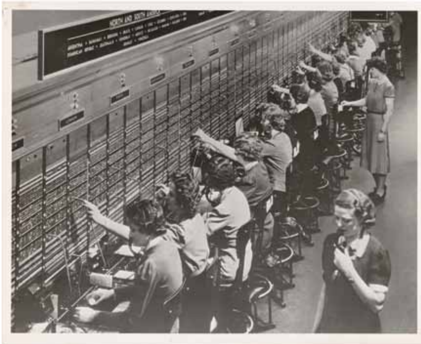
The source of the microphone plug used in civilian aircraft. This switchboard was typical of the tens of thousands such switchboards in common use by large companies from the 1920s through the 1950s.
