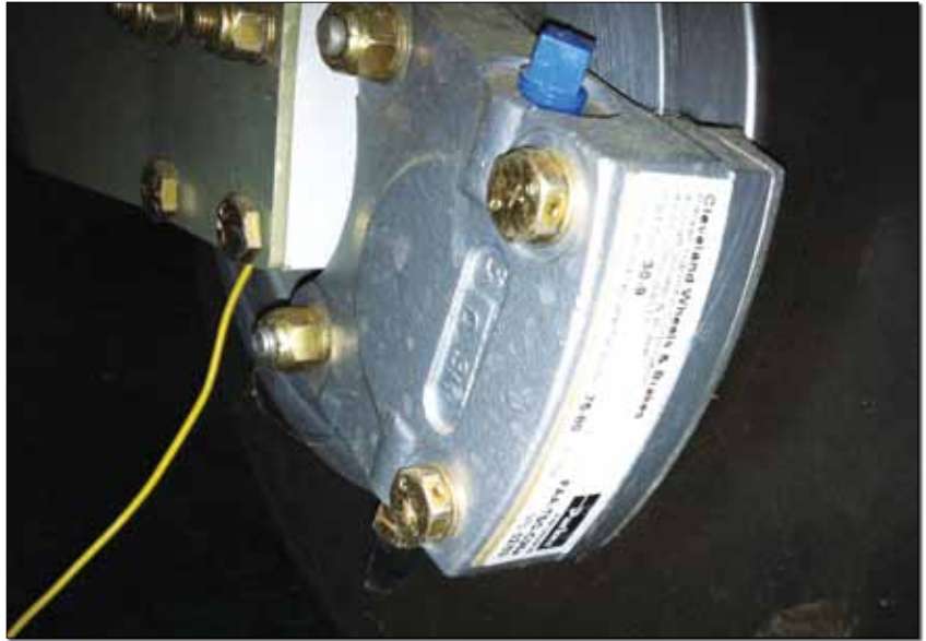
See the drilled holes in the bolt heads? These will require safety wire.
