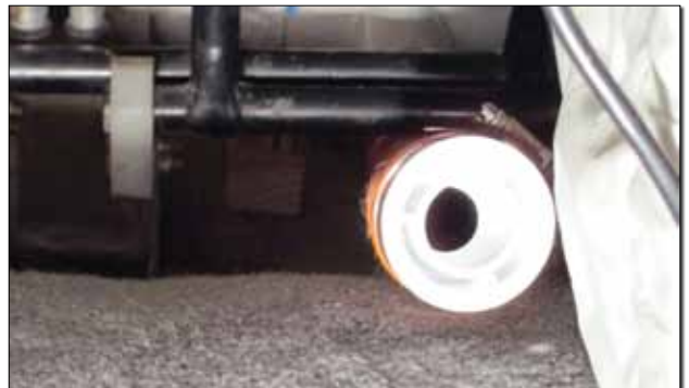
To increase the outlet pressure of cabin heat, PVC reducers were installed that decreased the outlet from 2 inches to 1 inch.
