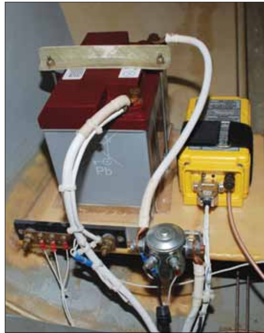
Make sure that all battery wires and terminals are clean and secure before worrying too much about your alternator. Note the ground bus bar in front of and below the battery. Good grounding eliminated many potential problems.
