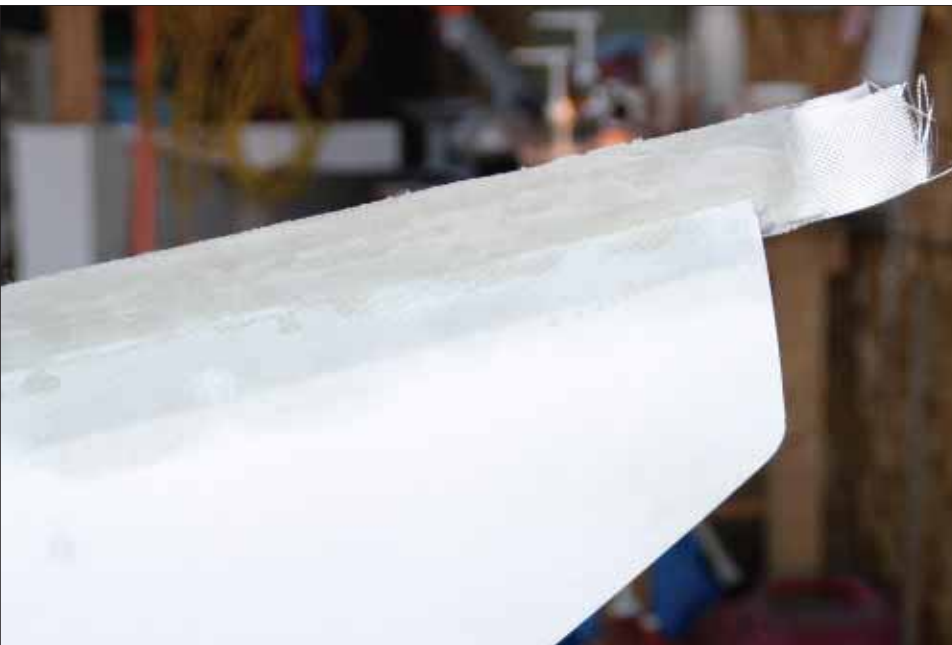
Several layers of glass extending beyond the needed zone gave the author more than enough to trim off with the saw.
